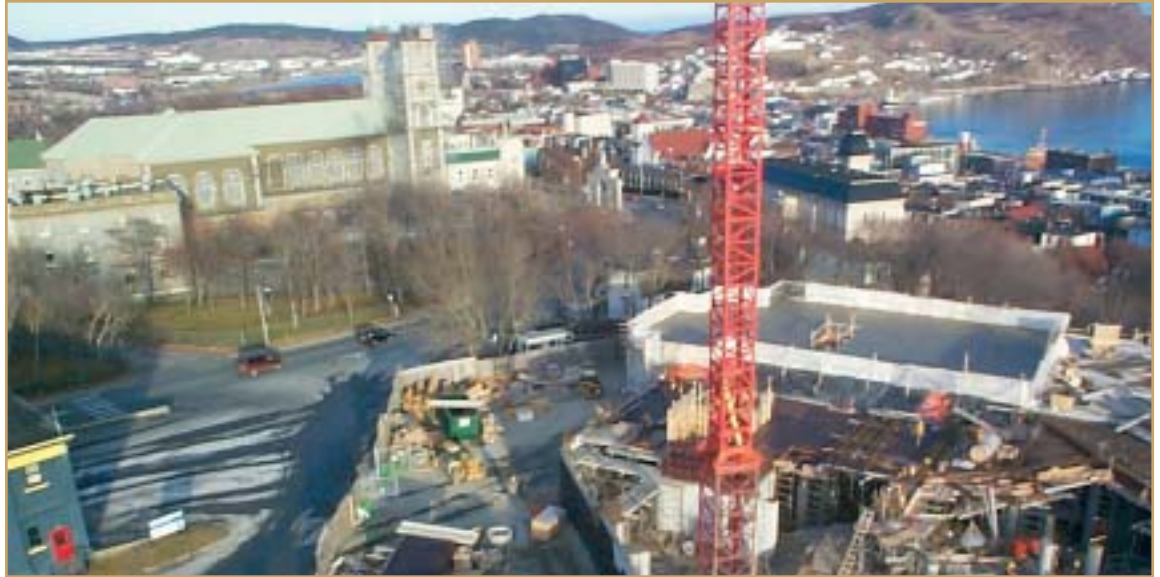
Credit: Provincial Archives of Newfoundland and Labrador Construction site of "The Rooms"
